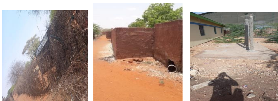
Figure 2-15: Wall and Bucket Latrine encroaching in Jogoo Location
