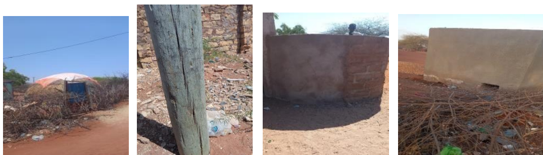
Figure 2-18: structures (hedge, power pole, fence and latrine) encroaching sanitary lanes in Wagberi Location.
