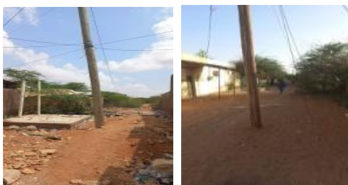
Figure 2-3: Septic tanks and KPLC power pole impacted in Township location
