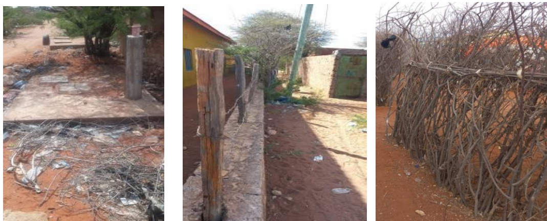
Figure 2-6: Structures (septic tank, fence, power pole and hedge) encroachment on the Sanitary Lanes in Hodhan location.
