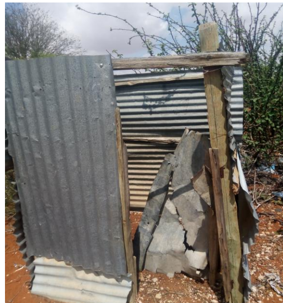
Plate 4-12: Pit Latrine with iron sheets without roof
