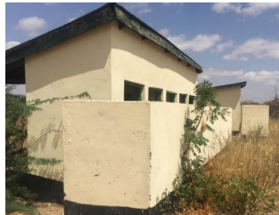
Figure 2-10: Existing Toilets in Furaha Mixed Secondary School
