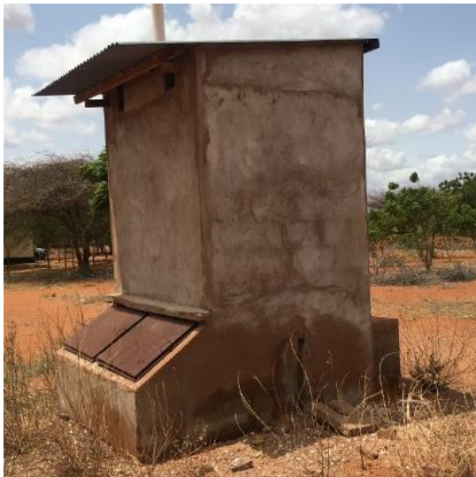
Figure 2-13: Ecosan Toilet at Wagberi Mixed Secondary School
