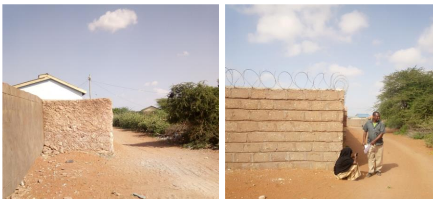
Figure 2-12: Masonry Walls encroachment in Godade location
