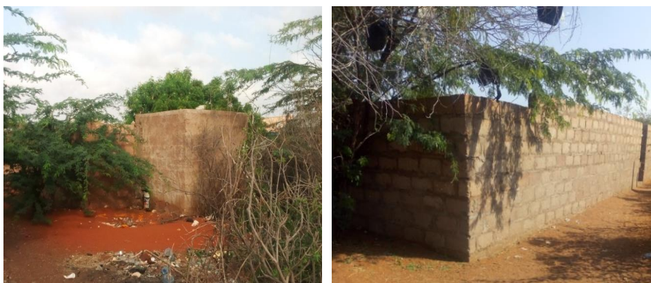
Figure 2-15: Wall and Bucket Latrine encroaching in Jogoo Location
