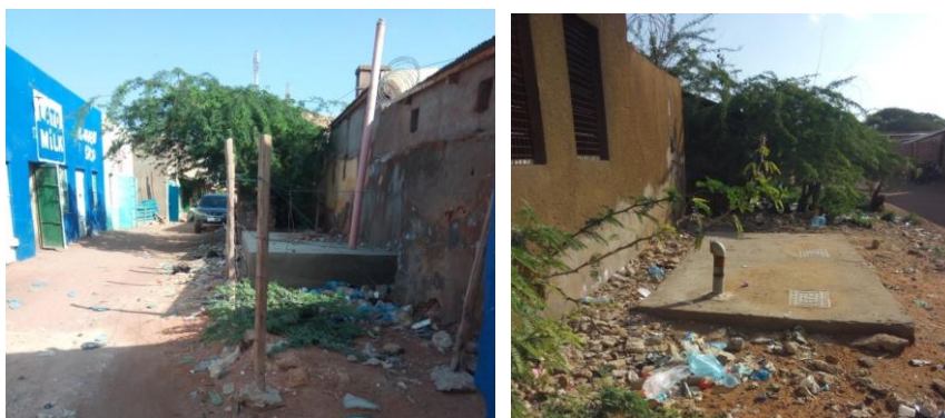
Figure 2-3: Septic tanks encroachment in Township location
